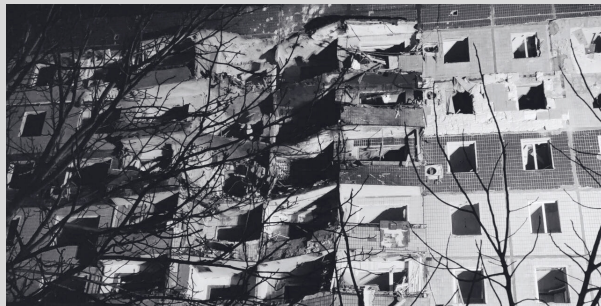
This 9-story apartment building was completely destroyed in the rocket attack.
