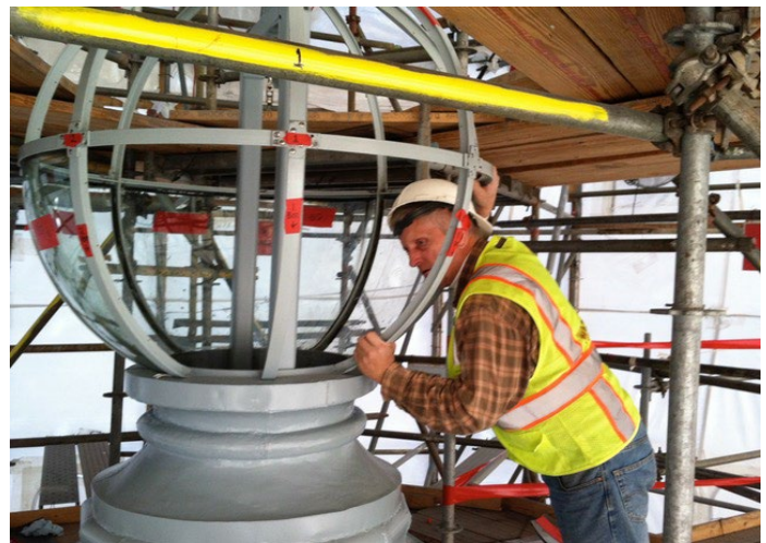
Phil Watkins working to restore the glass globe atop the Capitol building.
